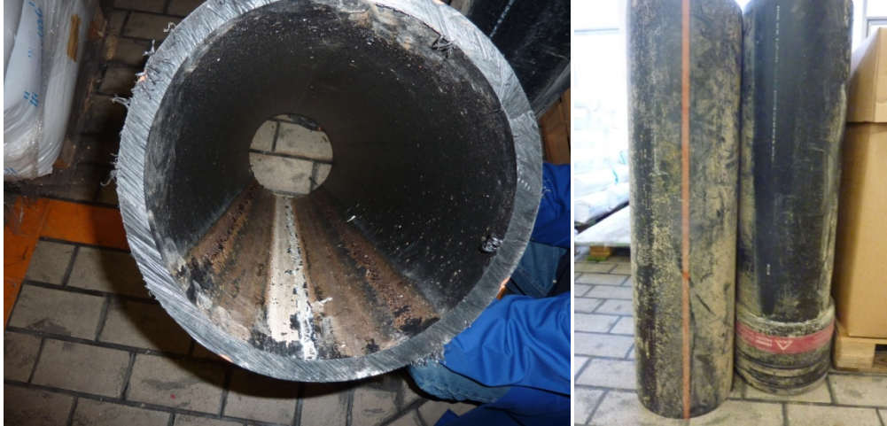
Figure 4.7 Black pipes with brown stripes, pipe G3
