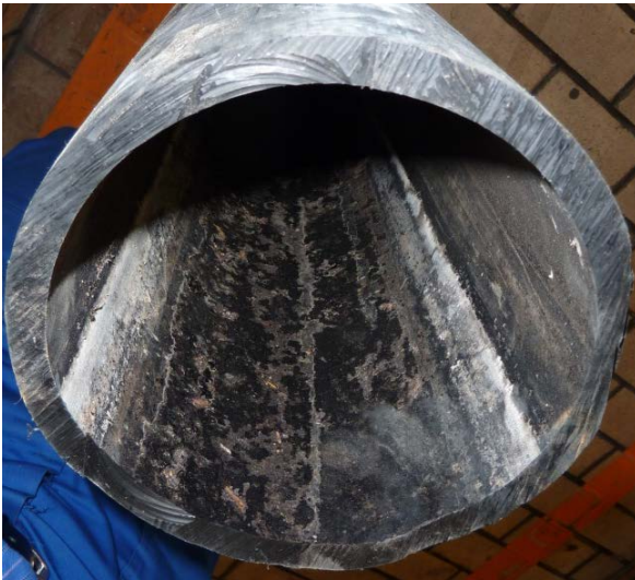
Figure 4.5 Deposits from waste water at the internal pipe surface marking the flooded area of the sewer pipe, F1
