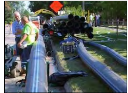
MID: HDPE water mains
