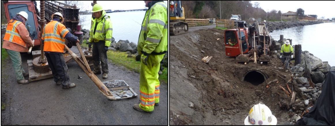
Figure 4. (Left) HDD battery powered locating sonde. (Right) HDD rig setup over existing host pipe.
