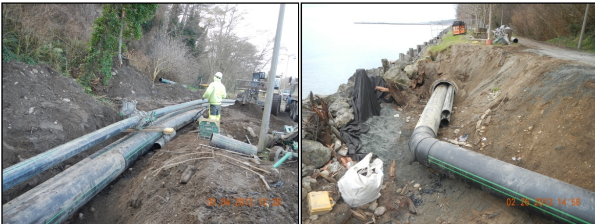
Figure 10. (Left) In-pit fusion of the 14-inch pipe. (Right) Fusion of the 30-inch pipe at an angle/elevation change.
