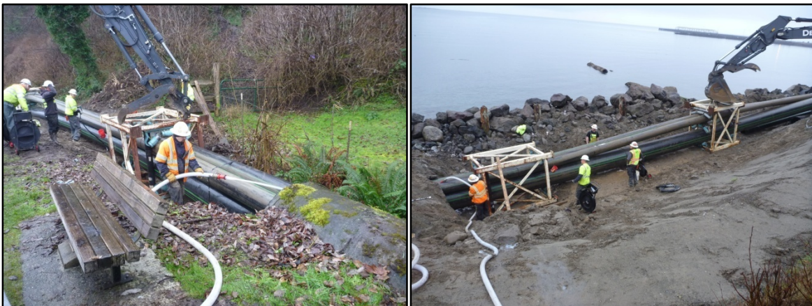
Figure 7. (Left) Pullback from pit C to B with liquid polymer lubricant. (Right) Pullback from pit F to D (see Fig. 3)
