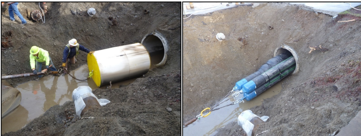
Figure 5. (Left) Proof and cleaning pig pulled prior to slipline. (Right) Test bundle pulled prior to slipline.
