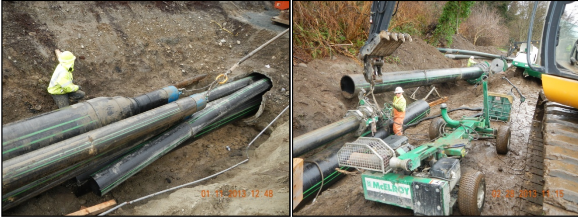
Figure 9. (Left) Slipline pit with two pipe bundles. (Right) In-pit HDPE fusion machines used to make connections.
