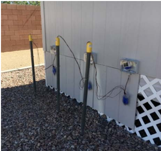
Figure A.6: Henderson, NV riser assembly (west facing)
