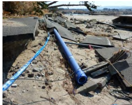
Pic2. Damage example (2)
