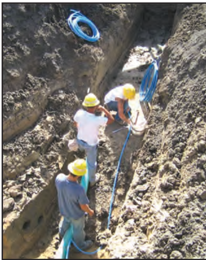
Figure 11.3 – PEX Water Service
