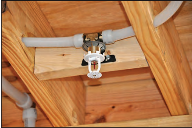
Figure 11.8 – Fire Sprinkler with PEX Piping
