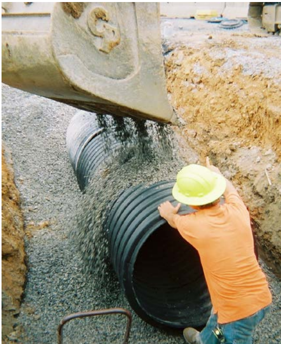
DICKSON COUNTY, Tenn. - Longitudinal installation of large diameter, corrugated high-density polyethylene (HDPE) pipe for storm water drainage systems was approved by the Tennessee DOT after a year-long, onsite study. The bed and backfill were properly compacted and followed standard industry practices, such as those contained in PPI technical bulletins and the PPI Corrugated Polyethylene Pipe Design Manual and Installation Guide.
