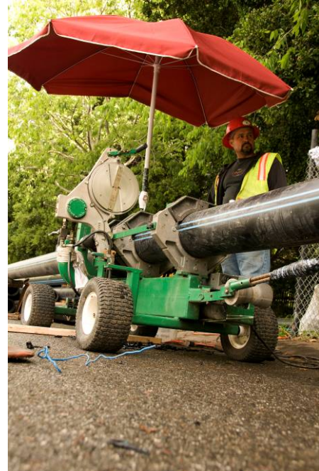
The majority of butt fusion was done on a McElroy Rolling 28 Combination Unit
