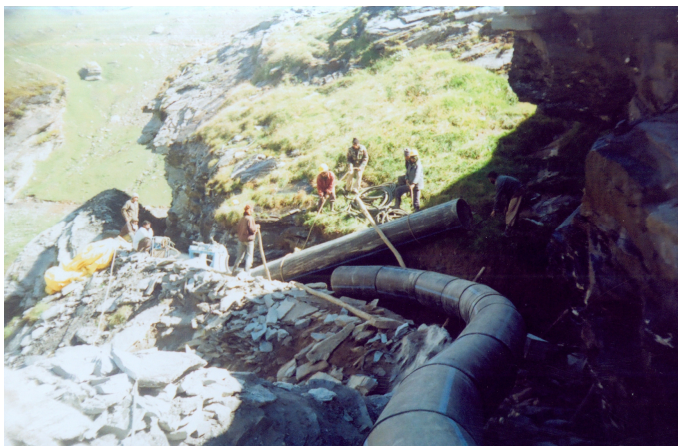
The ability of HDPE pipe to follow the contours of the land, have strong, leak-free, fused joints and be installed by a crew without heavy equipment was critical to the success of this project.
