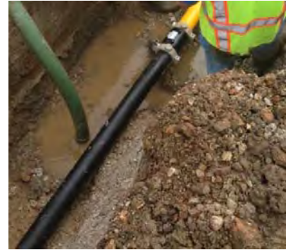
Figure I-a – Portable submersible pump (not visible)
