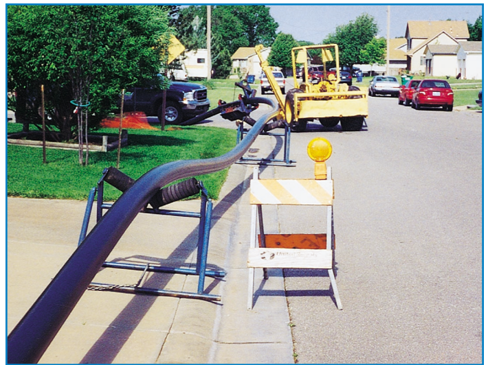
Fabricated unique custom rollers kept the pipe off the ground in areas where it might have been damaged during pull-back.
