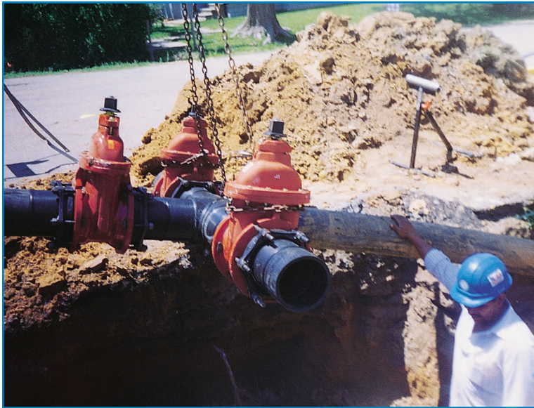
The project called for 97,000 feet of distribution lines, 108 fire hydrant assemblies, 804 service connections (not including schools) and more than 400 operating gate valves
