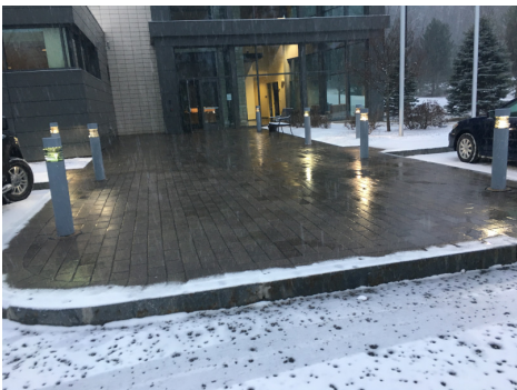
Hydronic snow and ice melting systems help keep outdoor surfaces clean during winter weather, while minimizing environmental impact.
