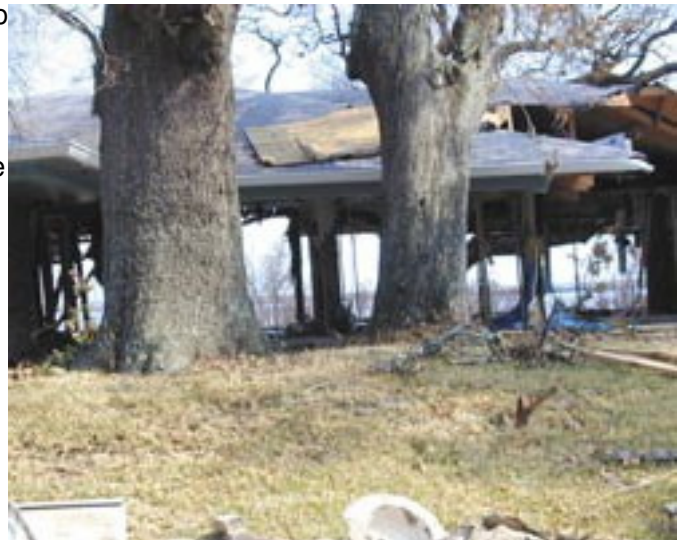
This was not built a pavilion. The storm ripped everything from this house but the support beams and roof.
