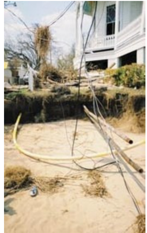
A close-up of the exposed pipes by the ruined beach-front house on page two. The PE gas pipe maintained its integrity. The sewer pipe, the water pipe, the house, and the land didn't.
