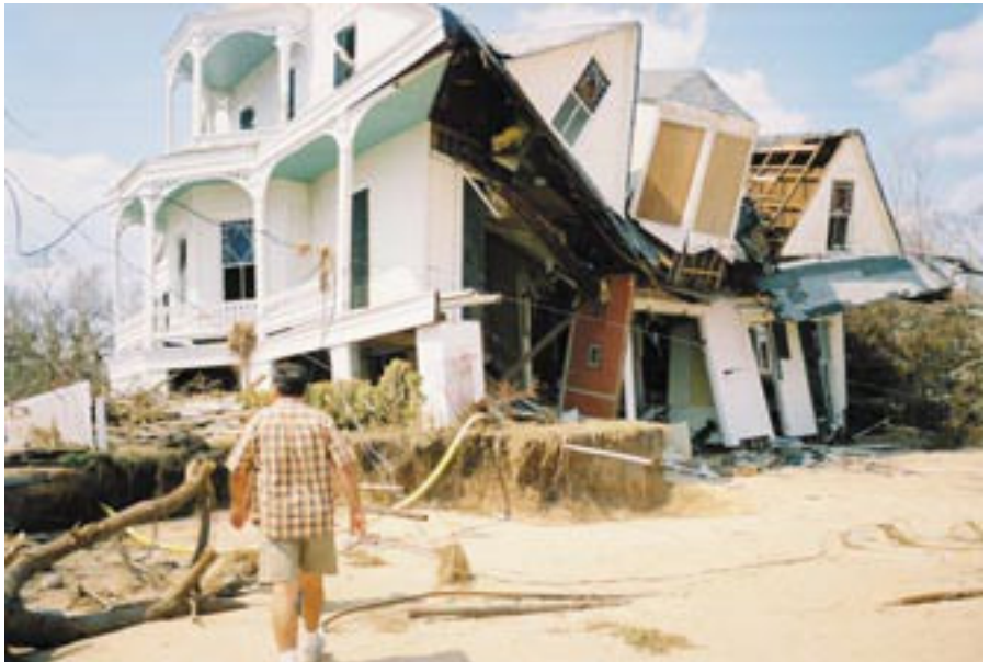
Buddy Zimmerman with Bay St. Louis, MS public works department walks towards the exposed gas lines in front of a ruined beach front house. This was a house that survived the massive Hurricane Camille in 1969...but not Katrina.
