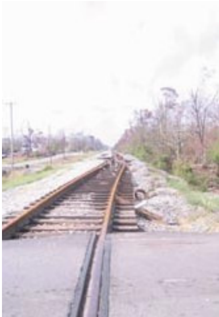
This is the railroad track that runs east-west through Waveland, Bay St. Louis, and other affected areas. It was the dividing line between the total destruction to the south (left), and damaged but often repairable to the north (right). The storm surge twisted the tracks. Look closely in the back, and you will see there is a house on the tracks that was washed off its foundation.
