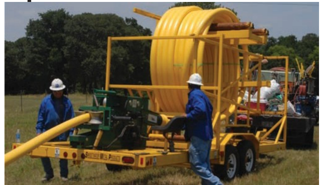
Medium Density Polyethylene pipe is used for gas lines. Coming on hundred-foot reels speeds installation for the crew.
