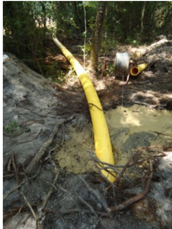
Installing the new 8-inch gas line using horizontal direction drilling (HDD) provided a quick, less disruptive installation of 93,000 feet of PE pipe.
