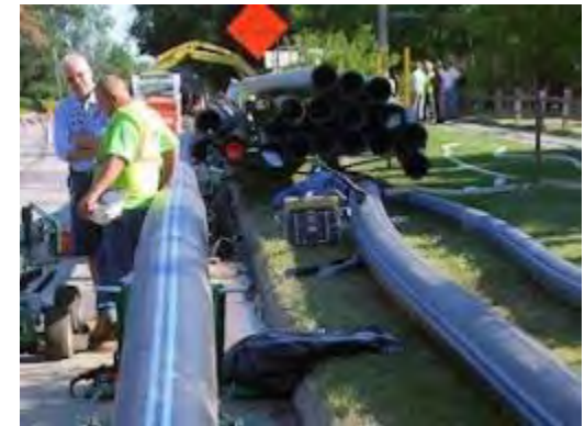
MID: HDPE water mains
