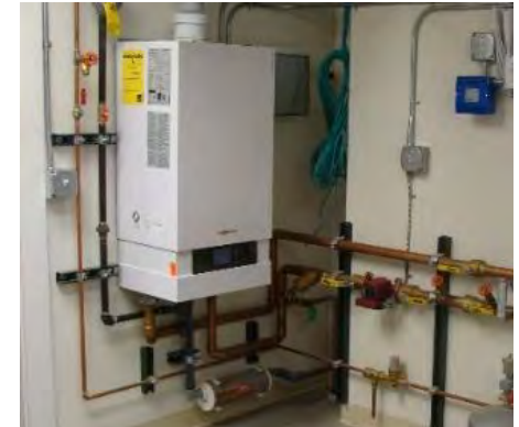
This system will use a dedicated boiler
