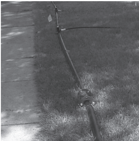
Figure 19 Example of Above Ground PE Bypass Pipe
