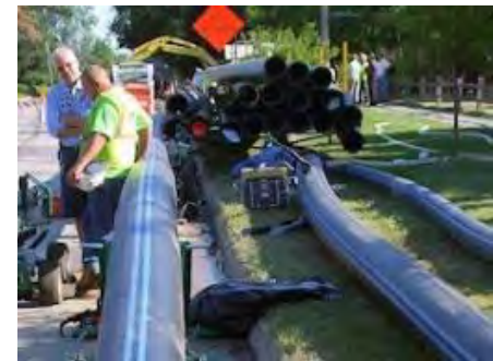
MID: HDPE water mains
