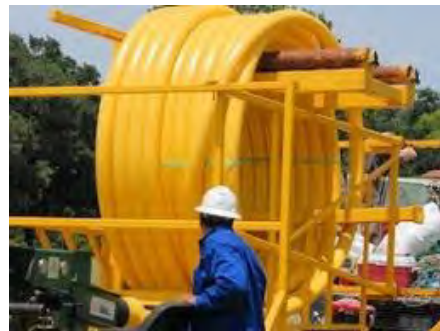
EPSP: Gas distribution piping
