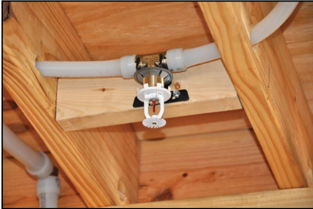
Figure 11.8 – Fire Sprinkler with PEX Piping
